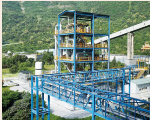
Taiwan's first power plant capturing CO 2 using the calcium looping method.
