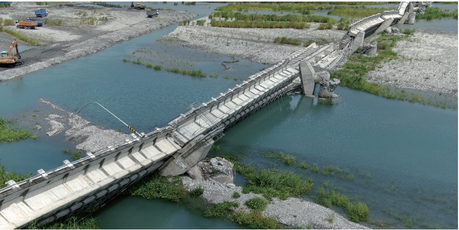
On Sep. 18, 2022, a 6.8 magnitude earthquake in Taiwan caused the Gaoliao Bridge in Hualien County to collapse.
